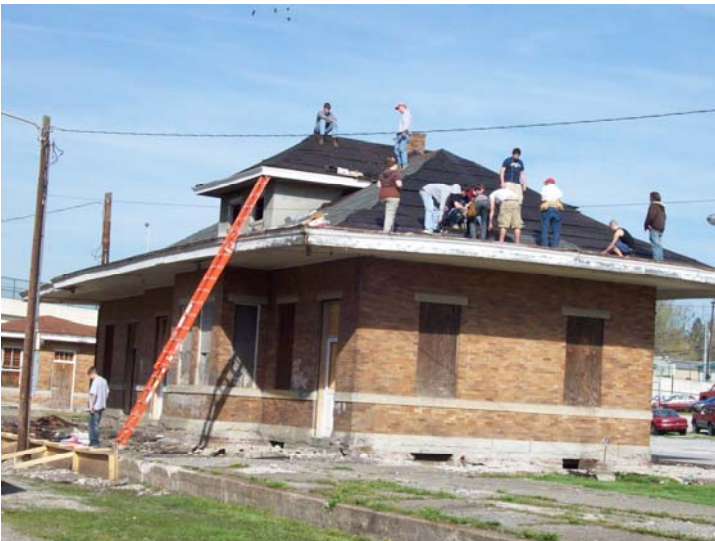
(Montgomery County Area Technology Students in Skills USA are restoring the roof of the Train Depot. The City of Mount Sterling received Transportation Enhancement Funds for the complete restoration of the depot by the Area Technology Students. Lynda Wilson, 4/2008)
